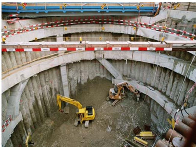
Fig. 5 Tunnel-gate shaft (see Fig. 4, section A–A'). The shaft reaches down to the bedrock
