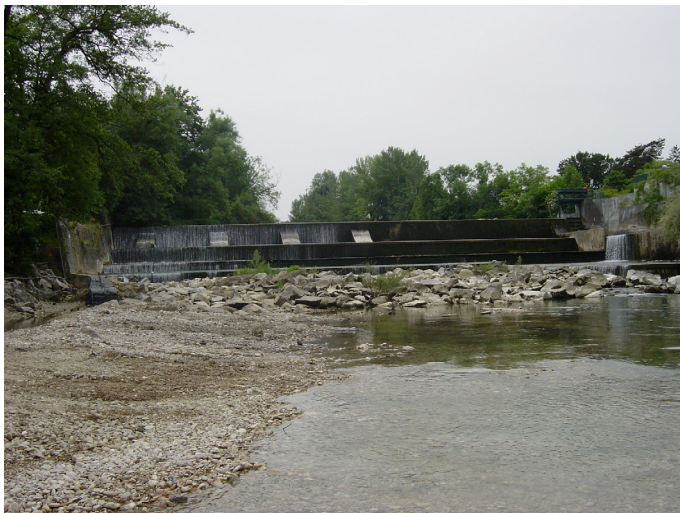
Fig. 4 River dam at low river discharge (9 m 3 /s; 16.06.2006). Note, as evidence for the subsidence of the dam structure, that the crest is only overflowed on its left side (a diagram is given in Fig. 2)
