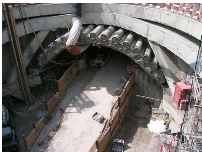
Fig. 6 From the tunnel-gate shaft the highway access and exit roads to the main tunnel are excavated using the “micropale” mining technique
