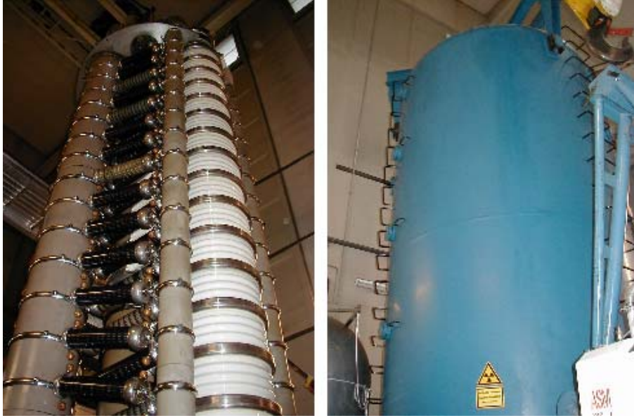
Figure 2.2: On the left picture one can see the high voltage cascade with the white porcelain acceleration tube and on the right the isolation tank of the accelerator.
