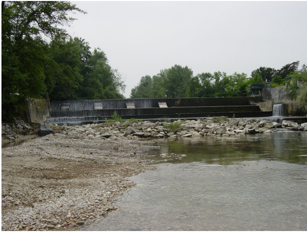
Fig. 4. River dam at low river discharge ( 9 \text{ m}^3 \text{ s}^{-1} ; 16 June 2006). Note, as evidence for the subsidence of the dam structure, that the crest is only overflowed on its left side (a diagram is given in Fig. 2).
